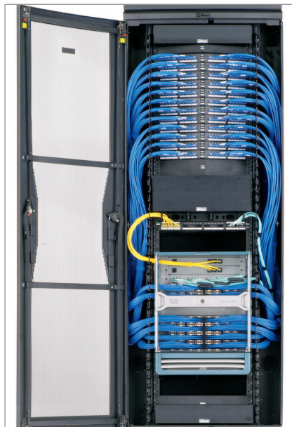
Single chassis in Net-Access™ Cabinet
